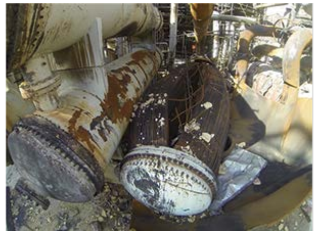
Figure 1. Post-blast photograph of the heat exchanger that ruptured catastrophically, causing extensive explosion and fire damage to the plant.
